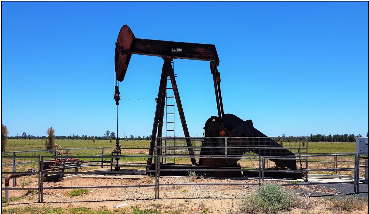
Moonie Injection Well 27 (M27)
