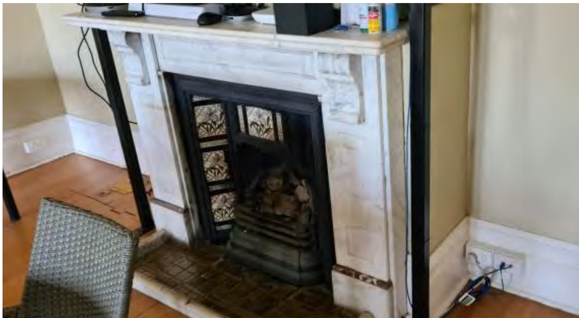
Internal views of fire places
