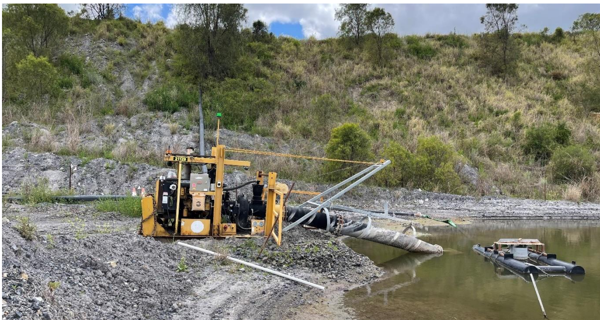
PHOTO 3: TYPICAL DECANT PUMP SET-UP
