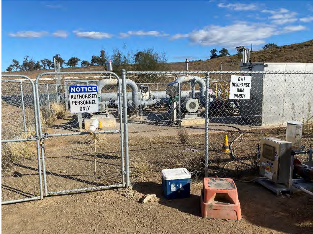
Plate 27 - Dirty Water Discharge Dam Pumping Facility
