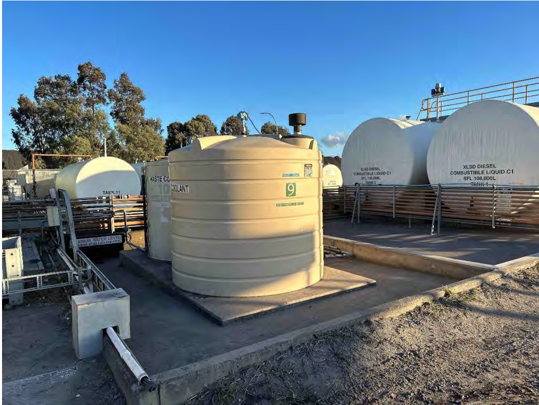
Plate 9 - Waste Coolant Tanks
