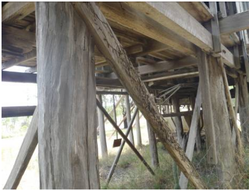
Photo 44 – Termite Tracks and Decay to Brace
