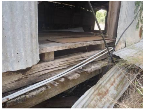
Photo 46 – Newer Floor over Old, Weathering & Decay of Old Exposed Members, Loose Iron Sheets
