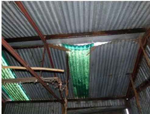
Photo 80 – Roof Battens Full Termite Attack, Completely Gone in Some Places – Sheeting has Collapsed Since 2011 Inspection
