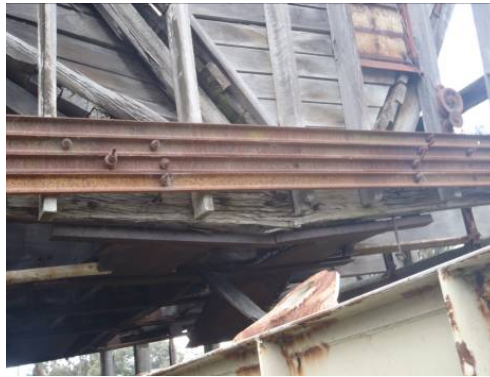
Photo 34 – Broken Hopper Joist, Railway Iron Strengthening
