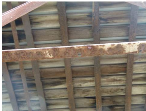
Photo 114 – High Level Bracing on Northern Side Rusted
