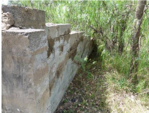
Photo 120 – Eastern Wall Cracked and Leaning Outward
