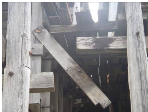
Photo 42 – Failed Joist Connection – Decayed Floor Boards
