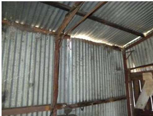
Photo 81 – Timber Top Plate Eaten Away by Termites in Workshop
