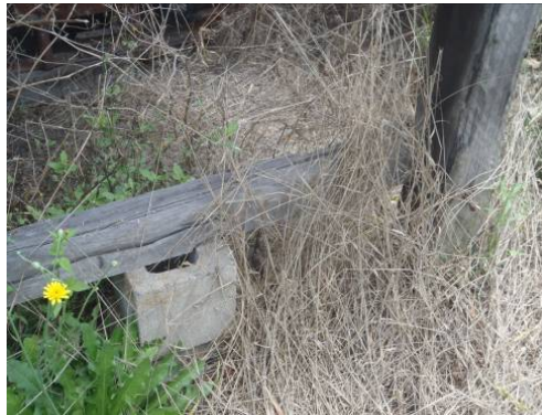
Photo 27 – Floor Bearer Propped on a Concrete Block
