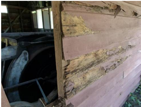
Photo 67 – Severe Termite Attack to Weather Boards
