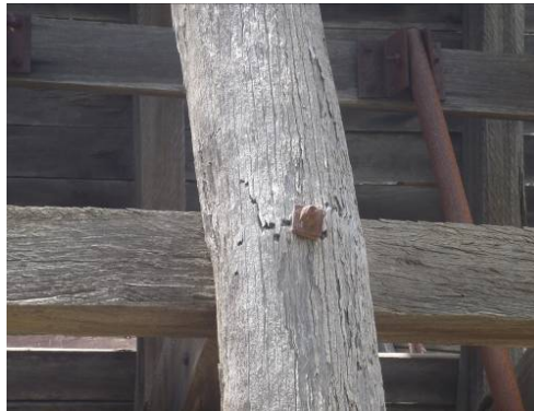
Photo 36 – Cracked Centre Support Pole to Hopper
