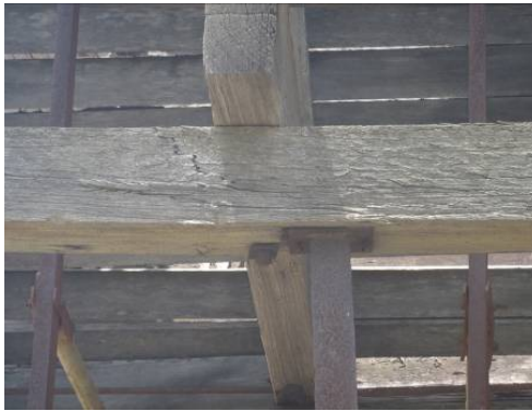
Photo 37 – Cracked Hopper Bearer at Steel Prop
