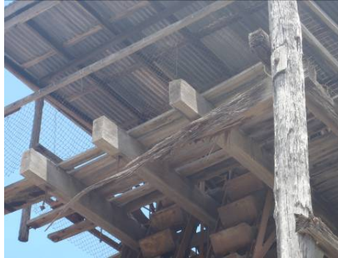
Photo 30 – Gantry Platform - Severely Decayed Bearer, Missing Joist
