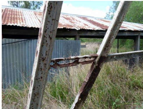
Photo 85 - -Lower Level Bracing on Northern Side Rusted
