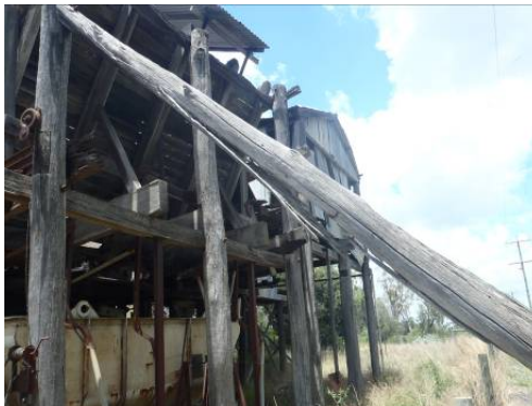
Photo 35 – Decay to Hopper Pole Props, Centre Pole Cracked, Bearer Cracked
