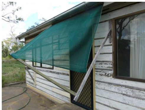
Photo 74 – Timber Awning Collapsed
