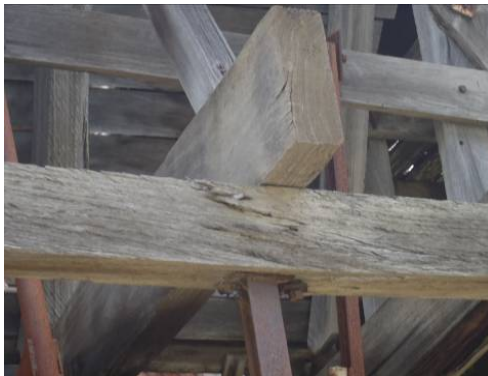
Photo 38 – Cracked Hopper Bearer at Steel Prop
