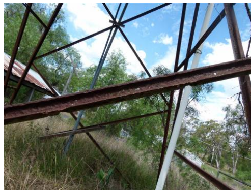
Photo 84 – Low Level Bracing on Western Side Rusted
