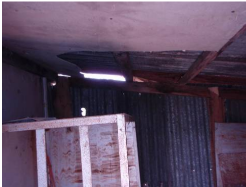
Photo 53 – Decayed Post and Roof Beam
