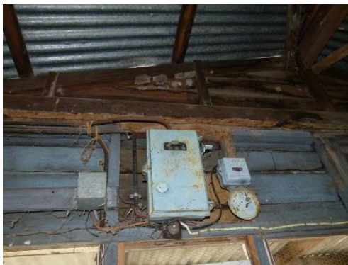
Photo 68 – Termite Attack to Underside of Roof Members
