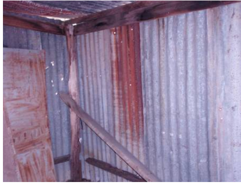
Photo 52 – Termite Damaged Post and Rail, Fallen Rafter
