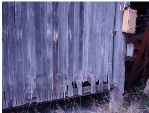
Photo 28 – Decayed Vertical Weatherboards to Picking Belt Shed
