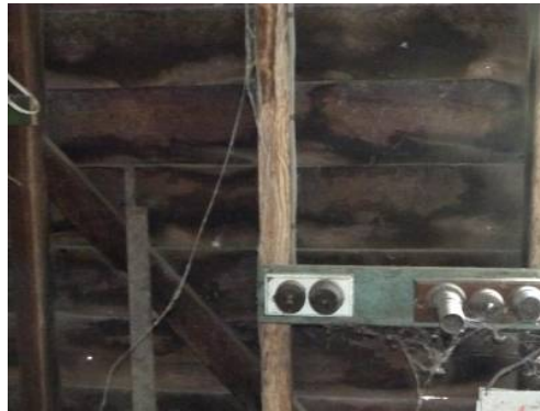
Photo 79 – Termite Damage to Wall Stud in Leccy shed
