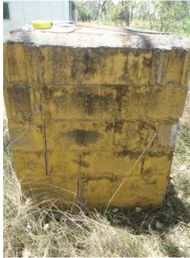
Photo 13 – Cracking to Wall
