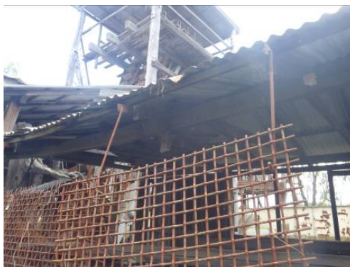
Photo 26 – Sagging Roof Beam
