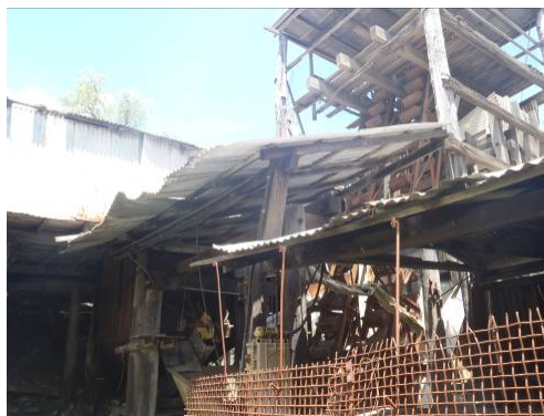
Photo 29 – Rotation of Post Extension to Lower Roof, Loose Roofing Iron
