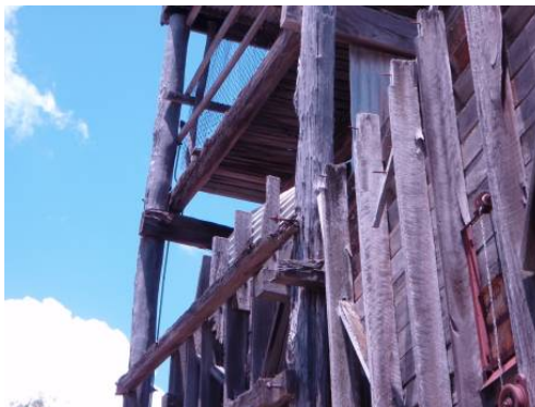
Photo 31 – Gantry - Decayed Exposed Members
