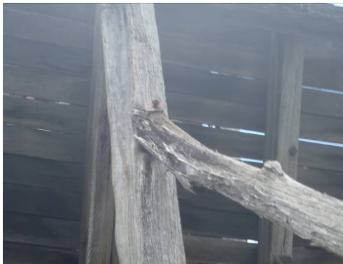
Photo 39 – Decayed Pole Prop
