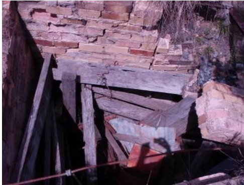
Photo 56 – Brick Walls Toppled, Timber Shoring
