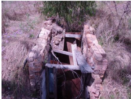
Photo 57 – Brick Walls Falling In, Timber Decaying
