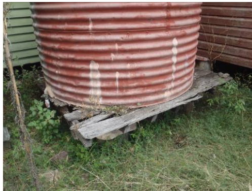
Photo 11 – Decay to Tank Stand
