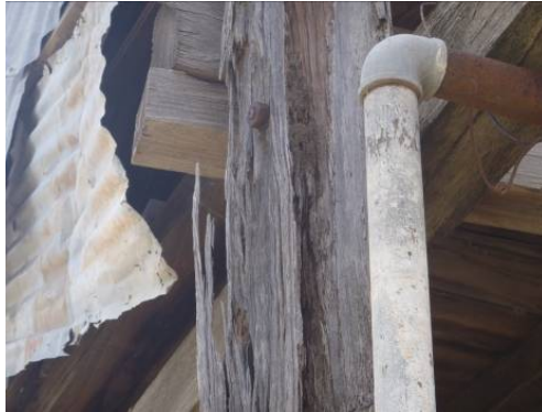
Photo 43 – Termites and Decay to Pole
