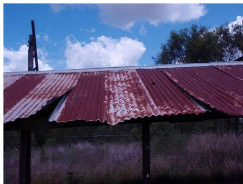
Photo 48 – Loose Roofing Sheets to Pit Head
