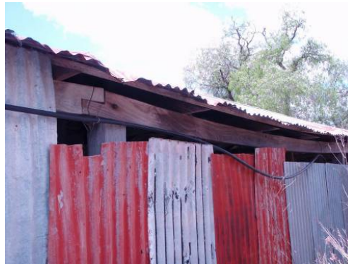
Photo 47 – Sagging Roof Beam
