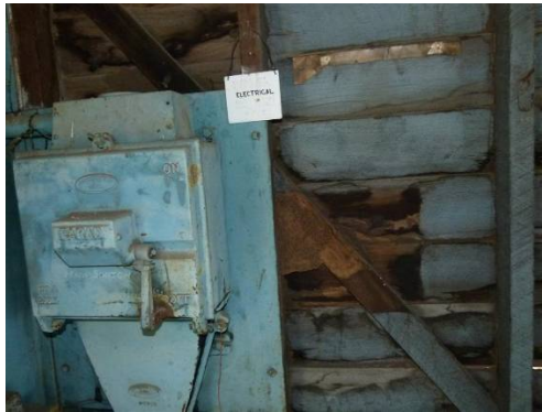
Photo 69 – Termite Nest on Eastern Wall Bracing Member
