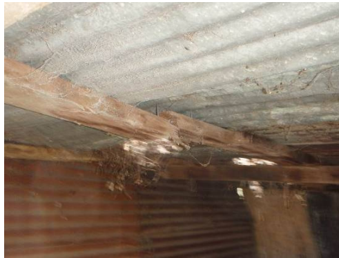
Photo 62 – Broken Purlin to Lean-to Storage
