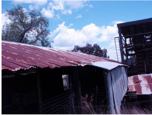
Photo 49 – Loose Roofing on Wall Sheets
