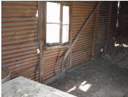
Photo 60 – Broken Stud with Termite Decay
