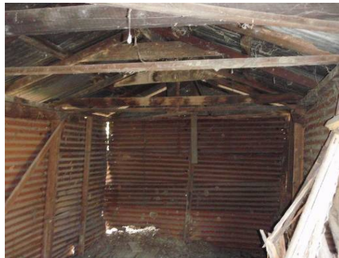
Photo 61 – Internal View Showing Broken Stud in Foreground
