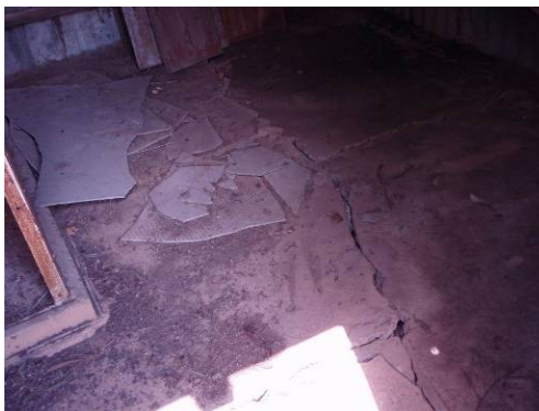
Photo 55 – Cracked Concrete Slab
