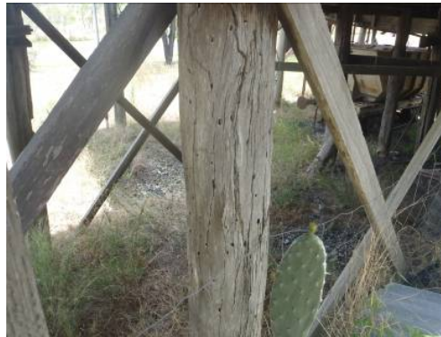
Photo 45 – Termite Tracks and Decay to Pole
