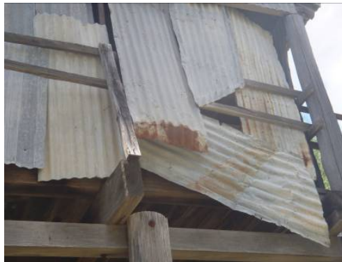
Photo 41 – Loose Sheets at West End of Pit Head
