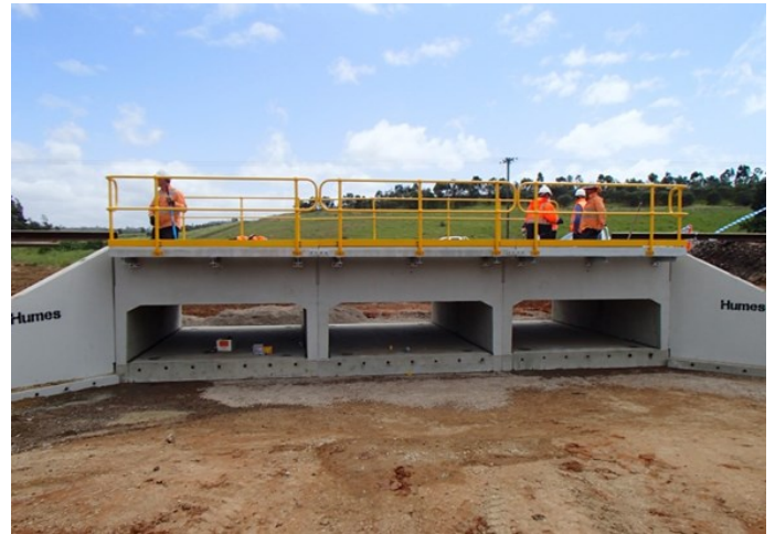
Installation of new culvert to ARTC rail lines during 62hr Shut Down
